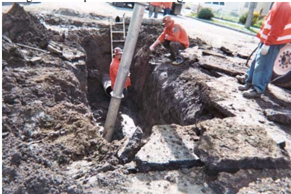
Saturday, February 26, 2011. 700 Block of Borregas water pipe blew out.
