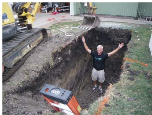
John stands in the hole where rain water will be stored in a cistern under the front yard.
