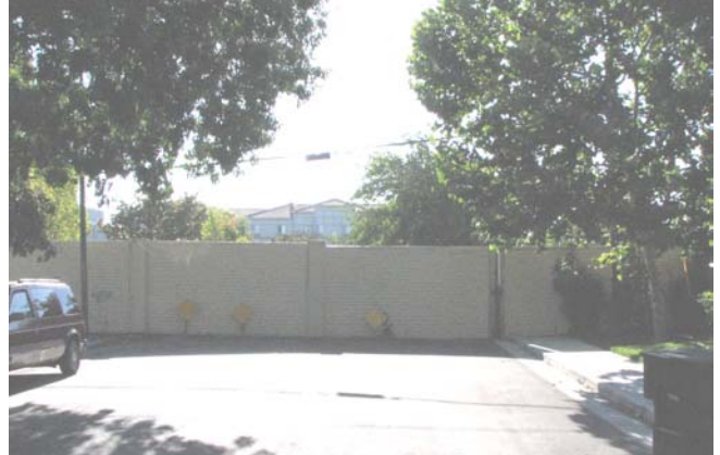
The threatened wall at the end of Ferndale Avenue.
