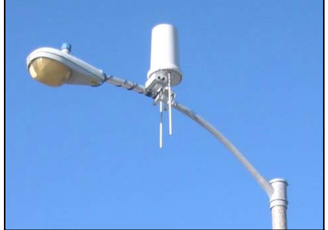
MetroFi Wireless Internet Access Point at the corner of West Arbor and Borregas.
